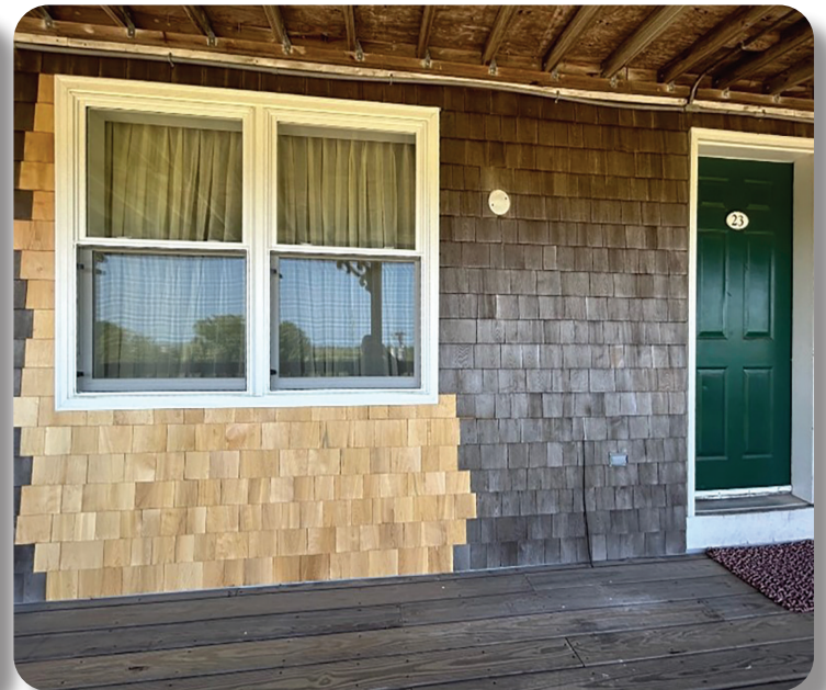
Framed-In Windows in Place of Sliding Glass Door
